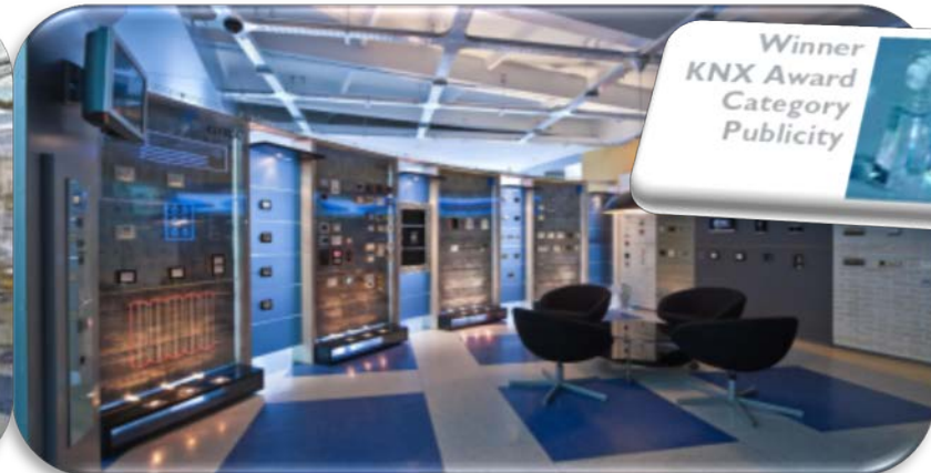
In the Showroom, display boards illustrate each of the different functions that are controlled via KNX
